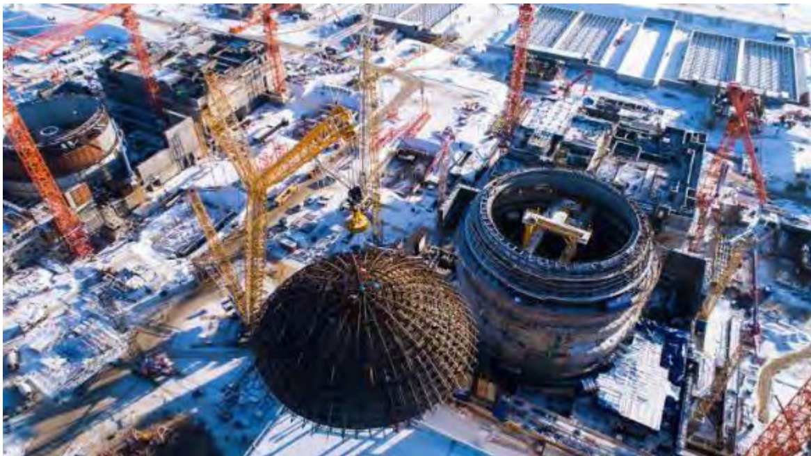
Kursk-II unit 2's The inner containment dome is hoisted into place (Image: Rosenergoatom)
