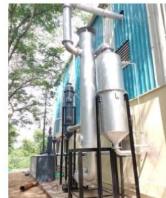
Heat exchanger, quencher and scrubber
